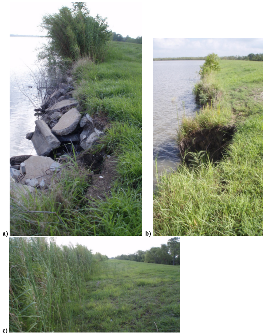
Figure 5.7. Pictures of Highlands Reservoir embankment levee. This includes (a) picture showing concrete rubble riprap and erosion, (b) unprotected embankment section with significant wave erosion, and (c) tall, dense reed growth that prevents inspection and provides burrowing habitat for animals. Images produced with permission from FNI and SJRA.
